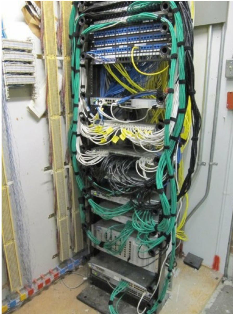
Figure 10.1 A typical wiring closet
